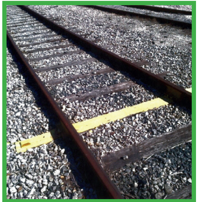
Markers to clearly identify the required holding position for parked wagons.
