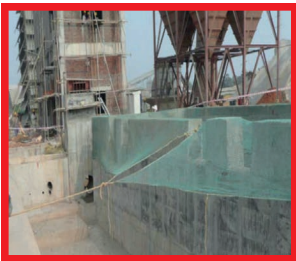
Fatal Accident 2011: Construction Project: contractor fell while crossing a wall during the construction of an extension.
