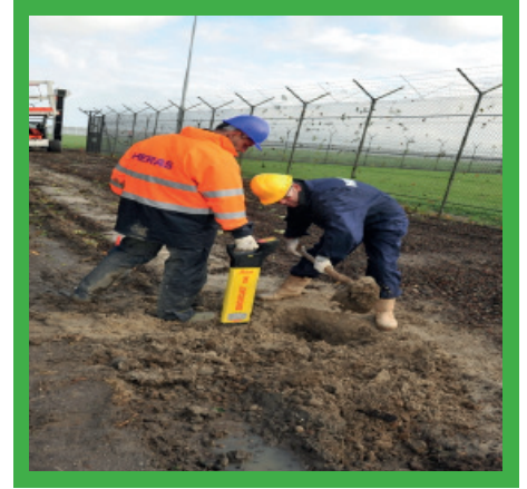
Checking for the presence of underground services prior to the erection of fencing.
