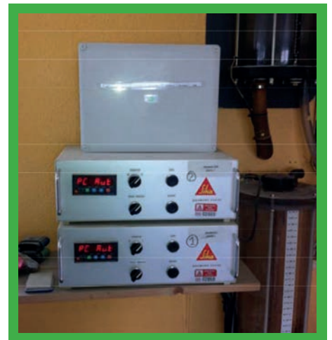
On site Receptor (top box).
