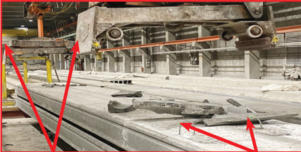
Hollowcore slab is lowered into position using the clamps / grabs from an overhead crane.
