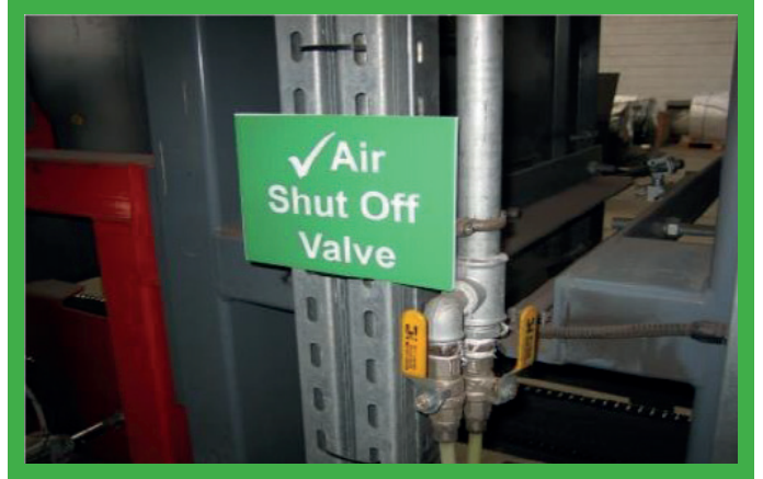
Clearly identified pneumatic isolation point.
