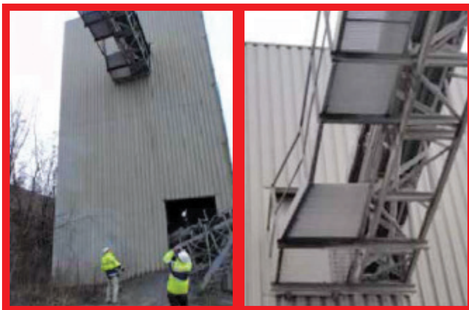
Fatal accident (non CRH site): Worker fell 14 metres when a section of walkway grid gave way. The grid securing bolts had become loose, over a period of time, due to the nearby vibrating screen.
